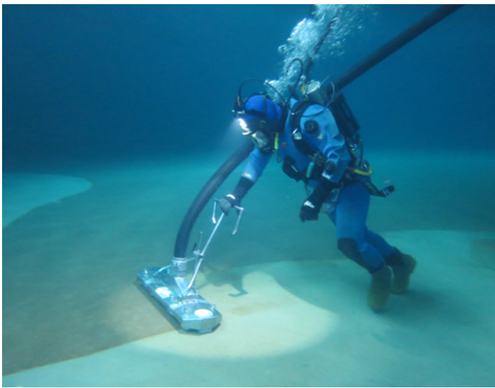
A diver vacuuming the bottom of a water storage tank. Note the highly modified vacuum head.
