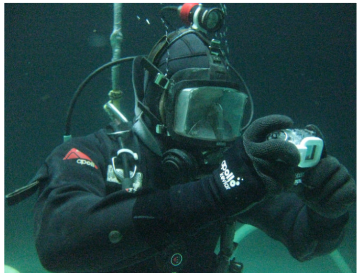
A diver photographing internal features of a water storage tank. Not the heavy thermal protection. Water temperature varies hugely depending on the location of the tank.
