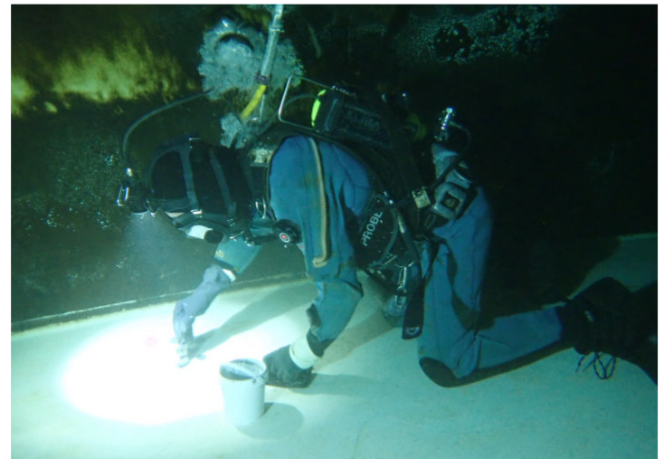
A diver repairing the floor of a water storage tank. Everything that is used in a water storage tank must be approved for use with potable water.
